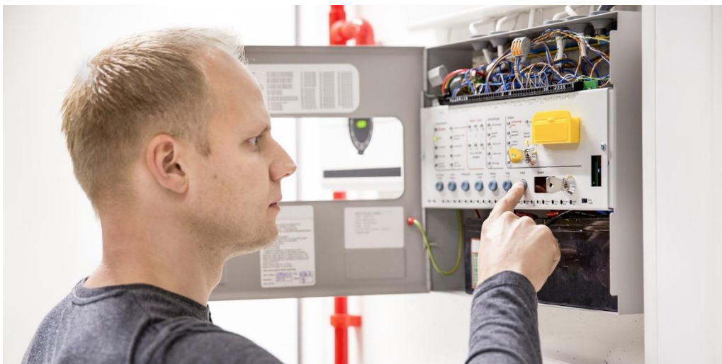
DTS Linear heat systems seamlessly integrate with fire control panel
