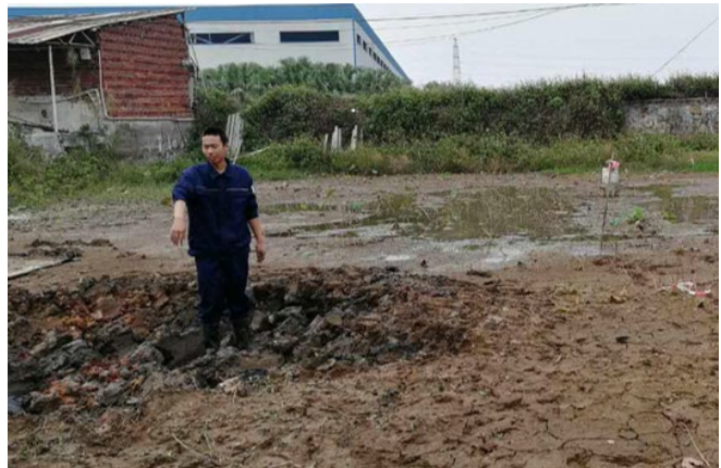
Photo of damage directly above pipeline
