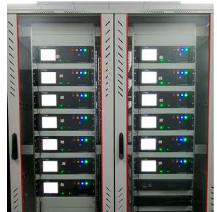
Figure 4: The 13 FireLaser DTS systems in the cabinet
