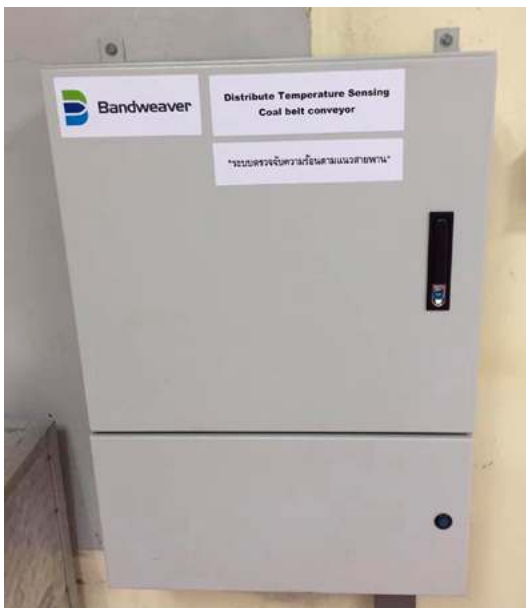
Figure 4: Wall Mounted FireLaser Installation
