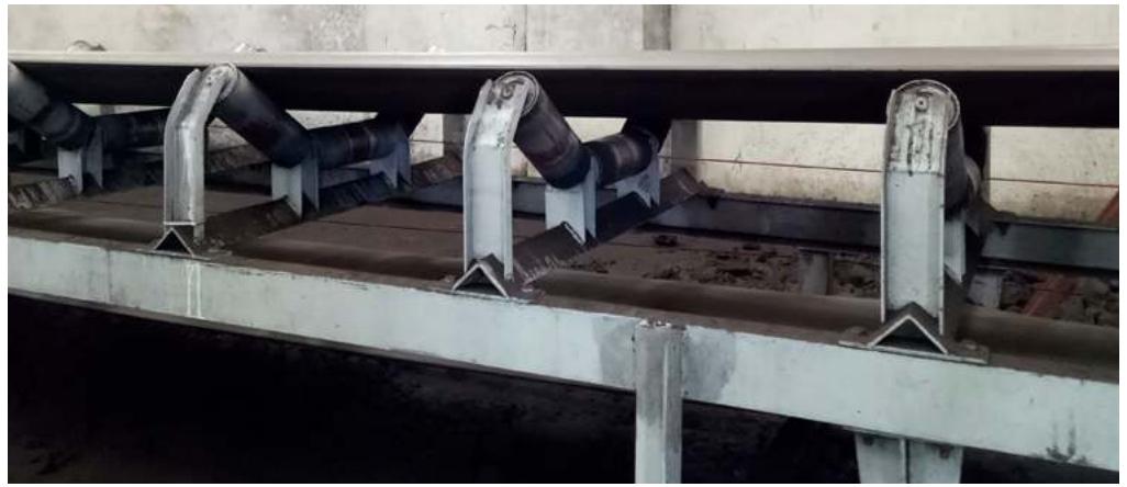
Figure 3: Cable route shown on conveyor belt
