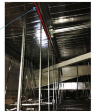
Fiber optic linear heat detection cable in ceiling void
