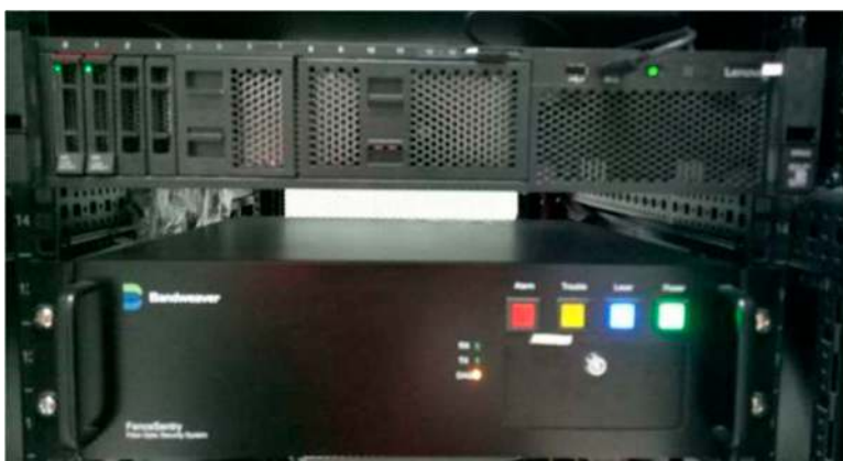
Figure 3 - Fence Sentry equipment installed in rack
