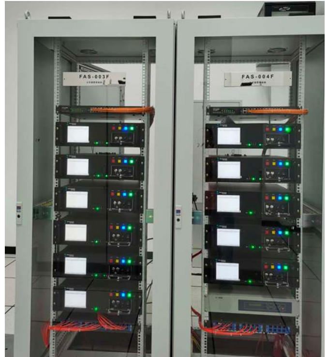
Figure 5: FireLaser LHD controllers in control room
