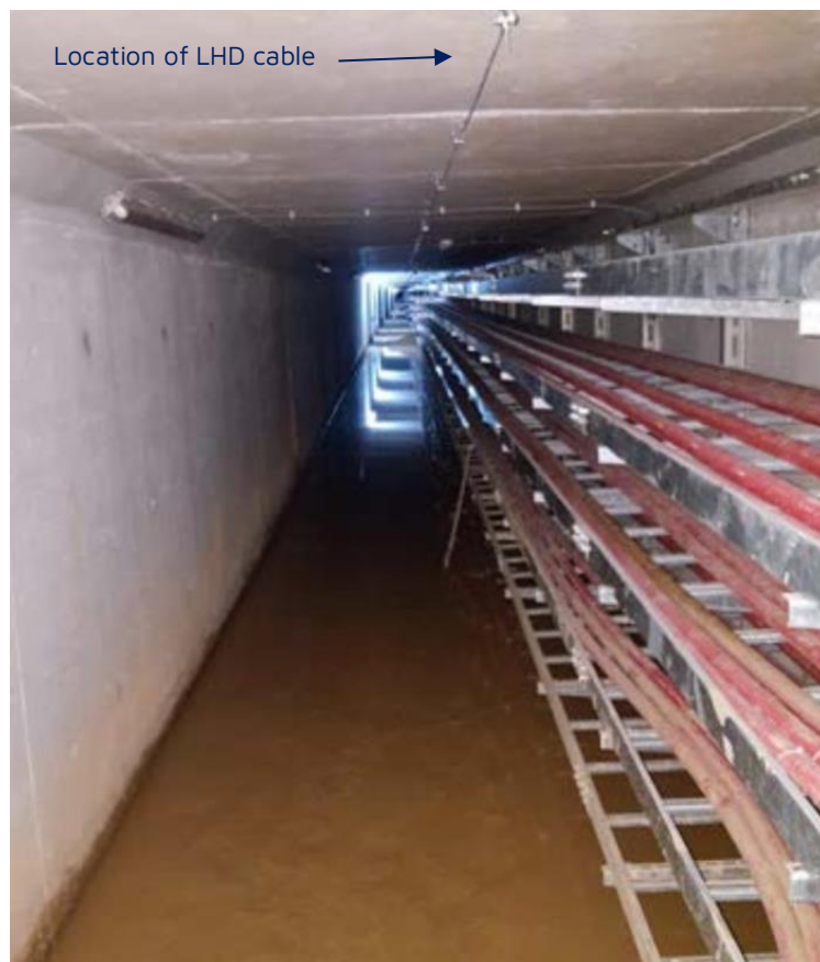
Figure 1 Photo of cable tunnel
