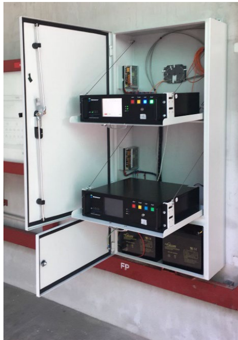
Figure 1 The dual system installed in the control room
