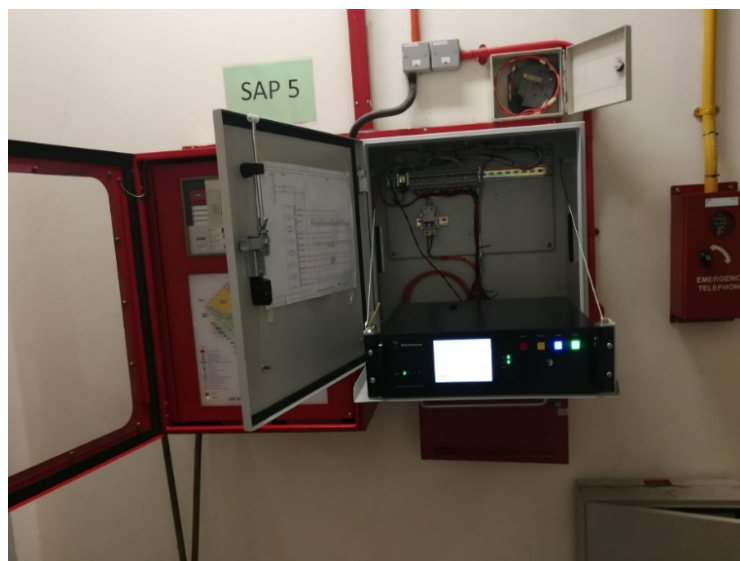
Figure 4 LHD panel and Fire Alarm Control Panel (FACP)
