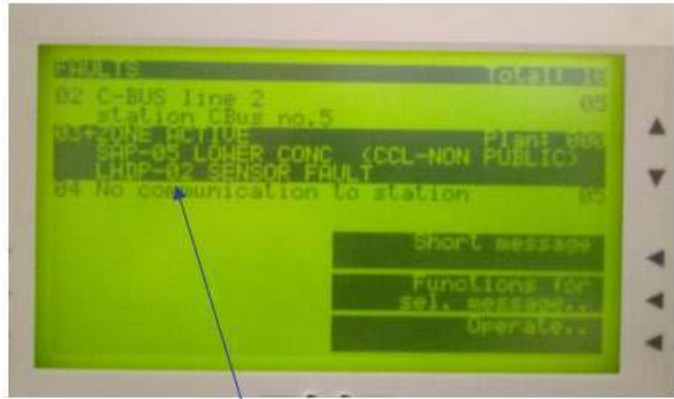
Corresponding system fault message on FACP
