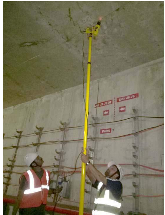
Figure 7 Testing the temperature alarms
