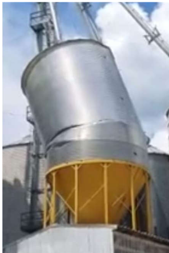
Figure 1 - Example of failed coil silo
