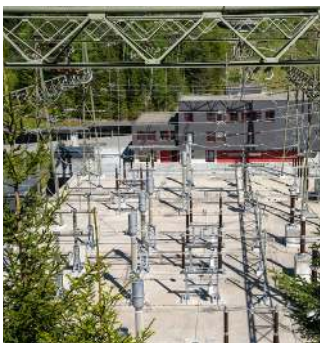
Power, utilities and substations
