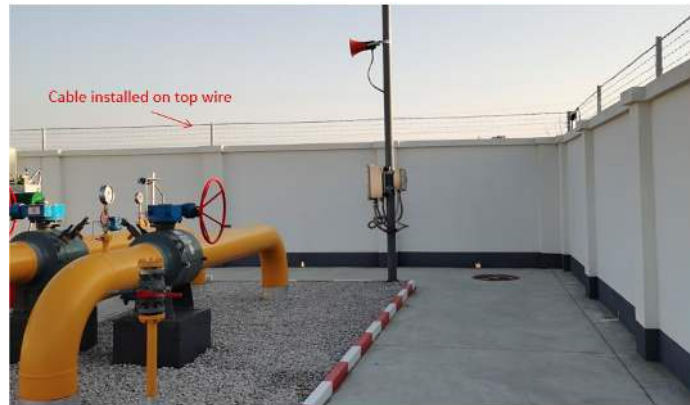
Figure 5 - Phot of cable mounted on fence topper section on top wire
