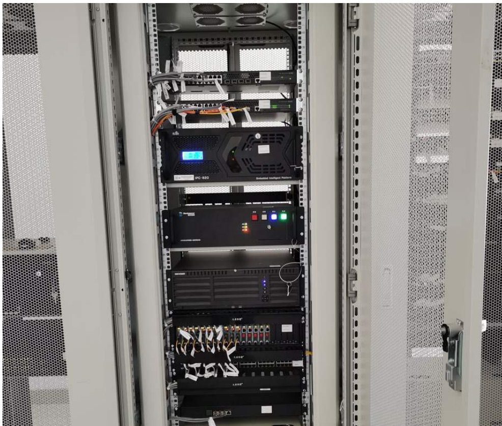
Figure 7 - FenceSentry installed in control room
