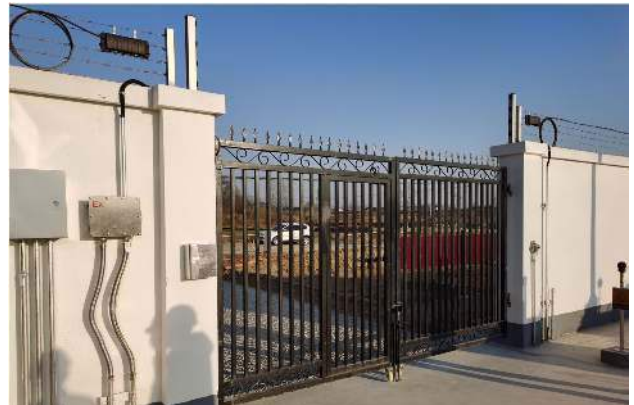
Figure 6 - Cable configuration at gate
