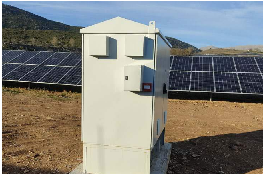
Figure 5 -Equipment enclosure cabinet
