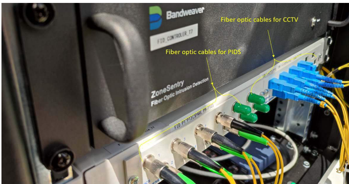
Figure 7 - Fiber optics PIDS and CCTV cabling within cabinet
