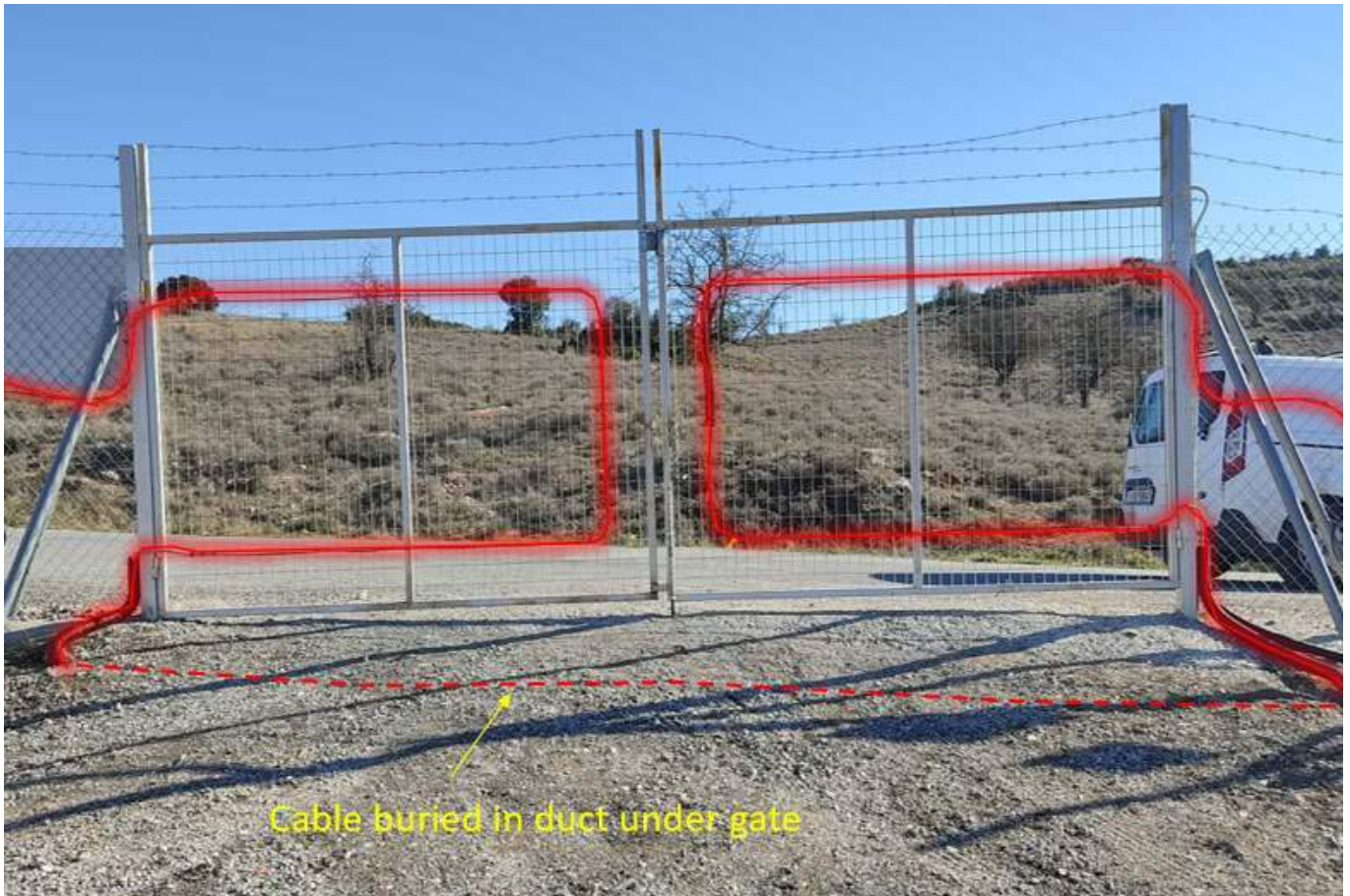
Figure 3 - Example of sensing cable installation on gate
