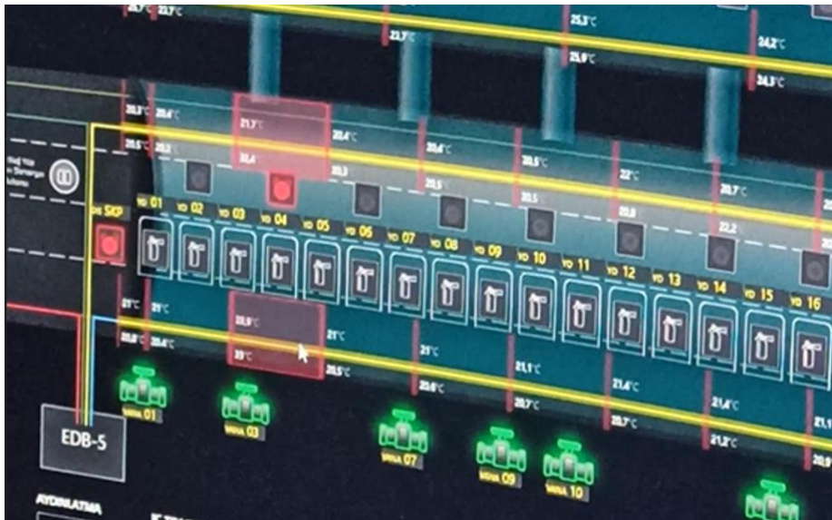
Figure 8 - Tunnel Management Software displaying alarm
