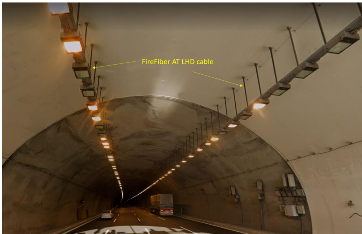
Figure 5 - Photo of FireFiber AT locations in tunnel
