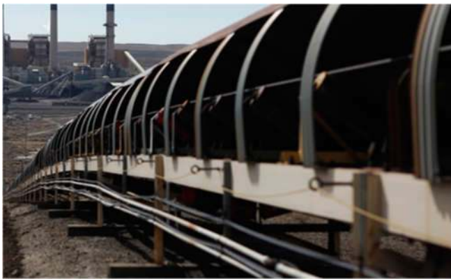
Conveyor to be monitored
