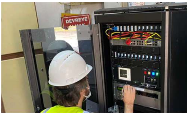
FireLaser LHD in instrument rack
