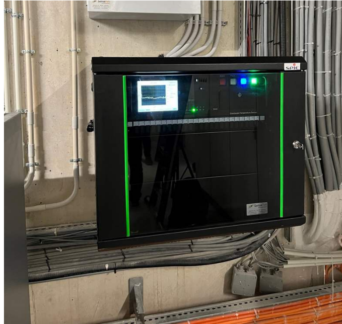
Figure 2. Example FireLaser system installed by SenseTek
