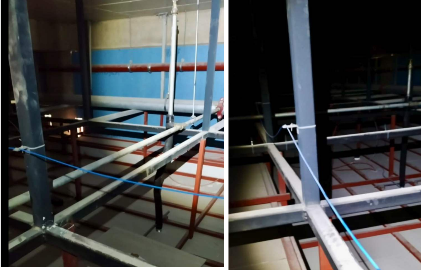
Figure 5 - Cable route in suspended ceiling
